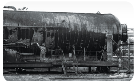
The damage sustained to infrastructure can be catastrophic during a fire event
