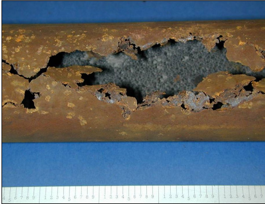
Figure 1. The air heater tube section in the as-received condition.
