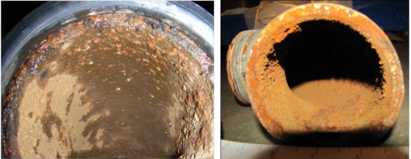
Figure 1. Examples of corrosion in galvanized piping in hot, softened water service.
