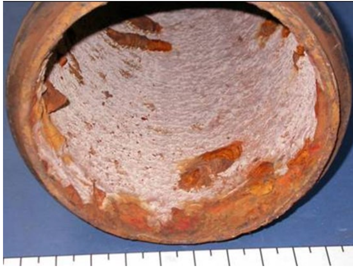
Figure 3. This galvanized pipe was examined after six years in service. This sample was from the cold, softened water line prior to the heat exchanger, but after the circulating hot water return. Pitting was significant.
