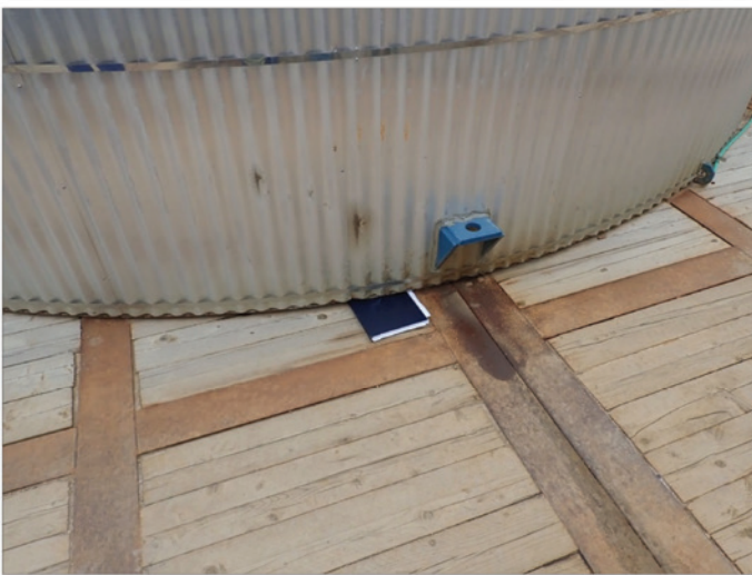
Figure 2. Gap between tank floor and supporting mat.
